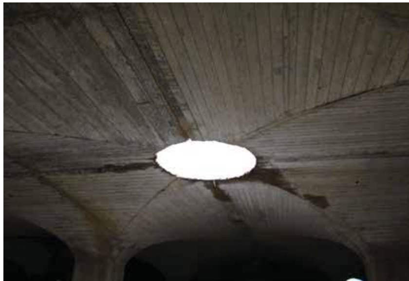
Manhole in Filter Bed 29. 2015.
