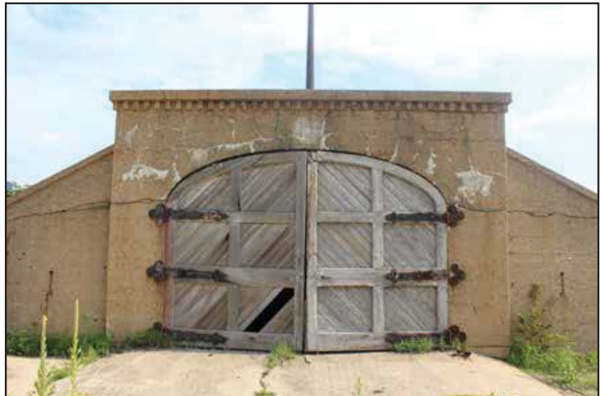
Filter Bed Portal 10, showing wood doors, hardware, and cracks along arch and walls. 2015.
