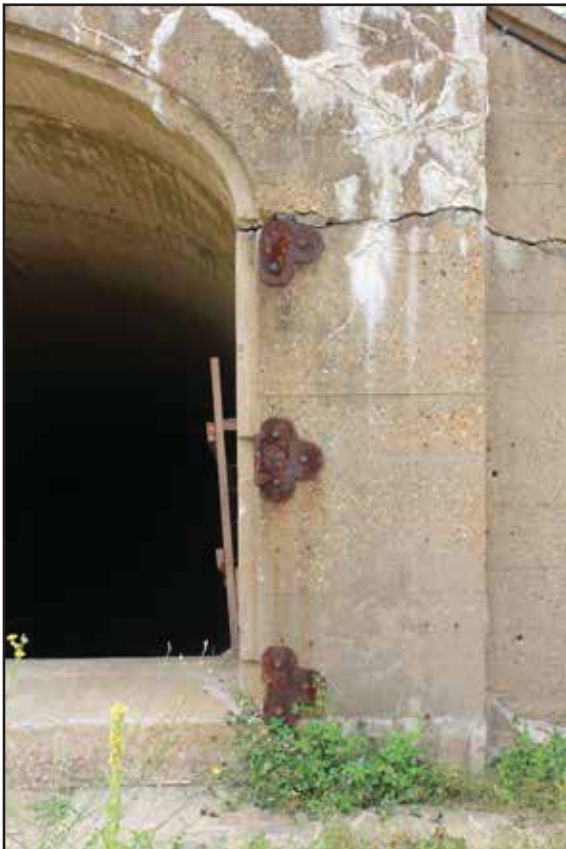
Crack at arch spring on Filter Bed Portal 15. 2015.
