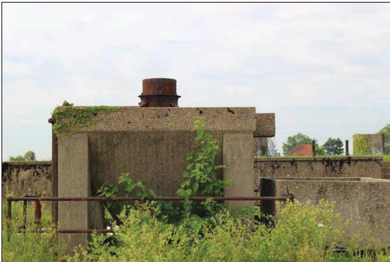
Sand washer 10 in Service Court 2, looking south. 2015.
