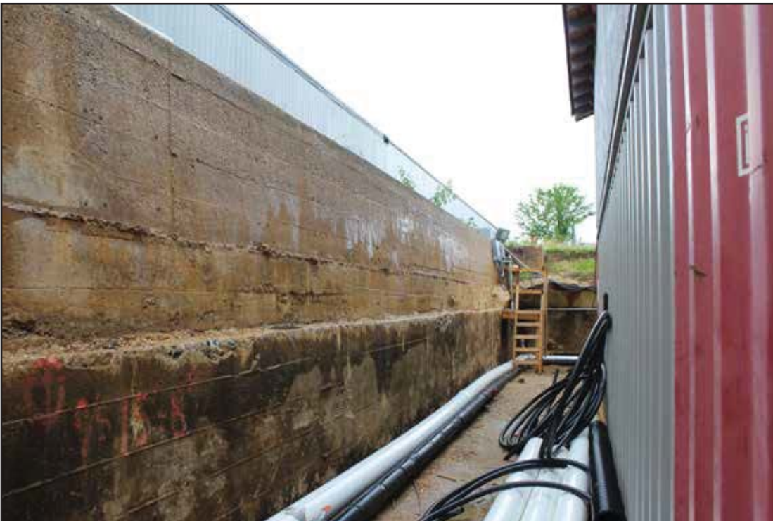
South Wall at Service Court 3, near Filter Bed. Looking northeast from south of the wall. 2015.
