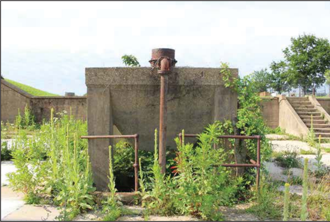
Sand washer 8 in Service Court 2, looking south. 2015.
